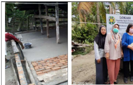
Figure 8.3. Repair of livestock shed floor and handover of PPE by USU Service Team
