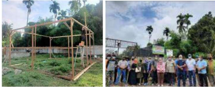
Figure 3.1. Construction of medicinal plant huts, collection of medicinal plants and completion of cottages collection of medicinal plants in Sei Semayang Village, Sunggal District, Deli Serdang Regency.
